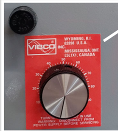
Variable Speed Motor Controller
